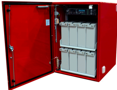
PS41-2730 Enclosure with (8) batteries and FXM650
