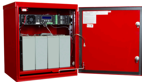
PS27-2220 Enclosure with (4) batteries and FXM350
