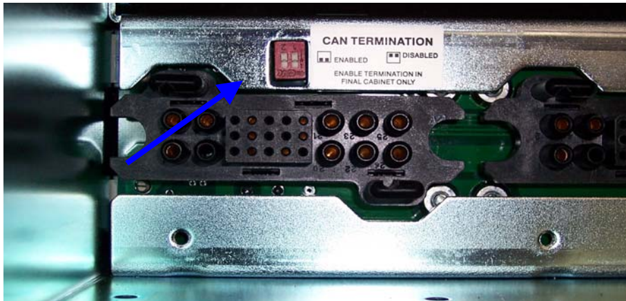
Location of CAN Bus Termination switches.
