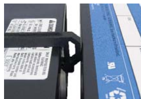
Detail of battery spacing
