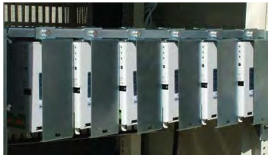
Figure 18–Six rack mounted FMPS power modules
