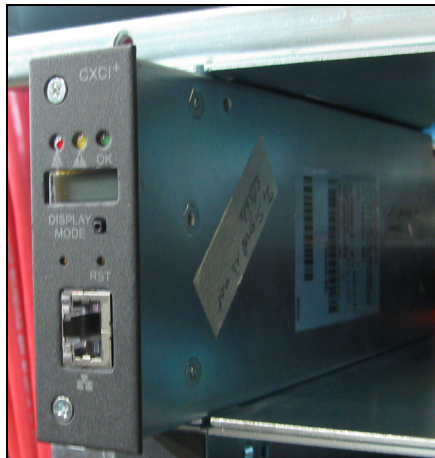
Figure 10–Showing CXCI+ controller module replacement
