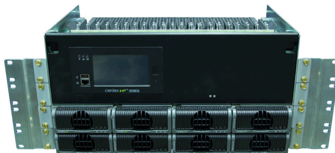
Figure 2 — Typical 48V Power System with 2.4kW Rectifiers
